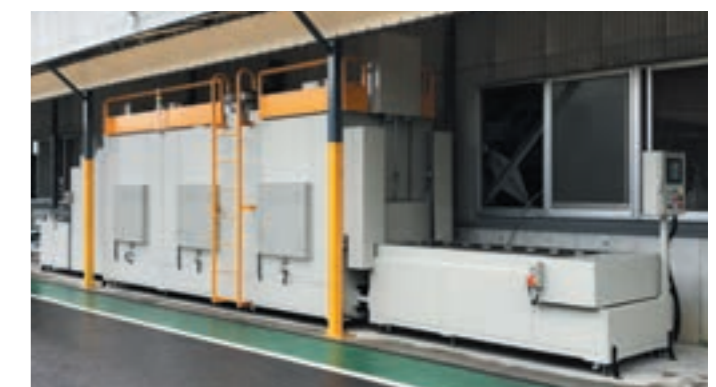
熱処理炉 Heat Treatment Furnace
